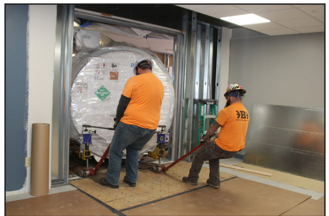
Crews attached a skate system to the bottom of the magnet which allowed them to roll the four-ton unit into the facility.
